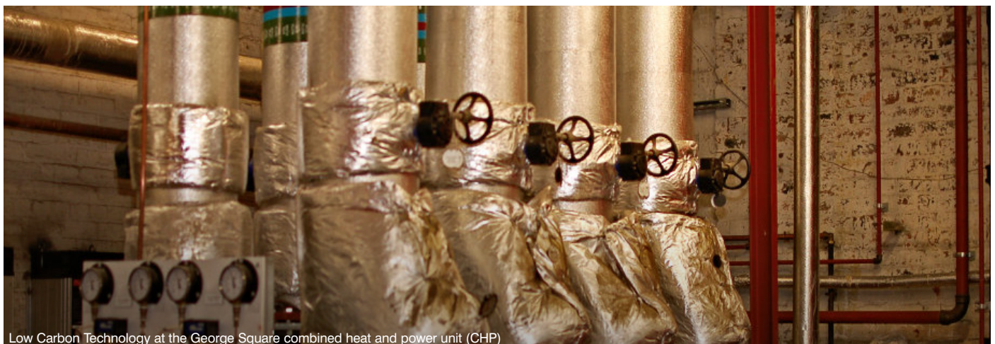
Low Carbon Technology at the George Square combined heat and power unit (CHP)
